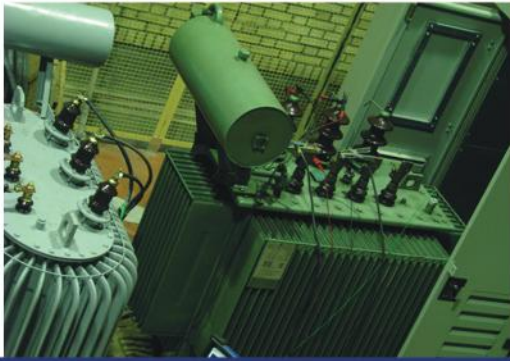
Switchgears, Compact Substations and Busbars Lab
